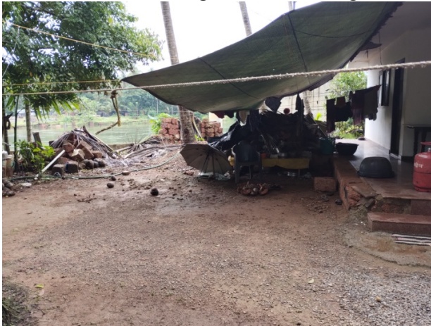
Affected Huse due the Piling work
