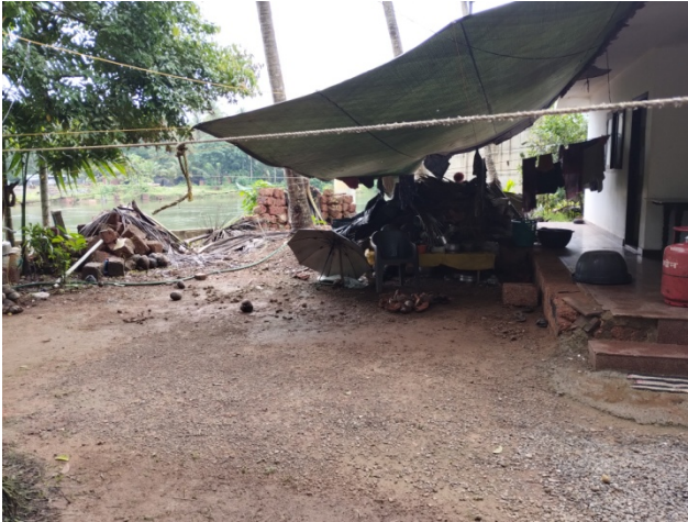
Affected Huse due the Piling work
